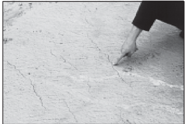
Plastic Shrinkage Cracks
